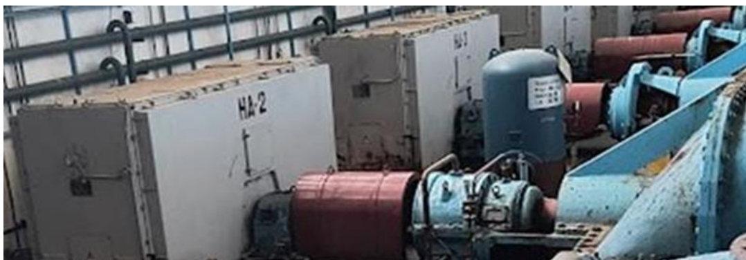
Figure 3-5 Old pumping unit with sliding bearings
