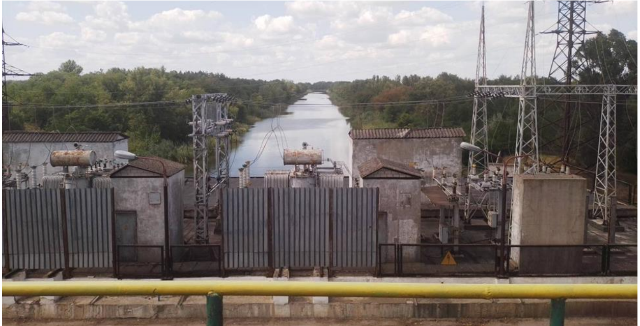
Figure 3-1 Obsolete transformers and main power equipment at the Dnipro-Donbass Channel
