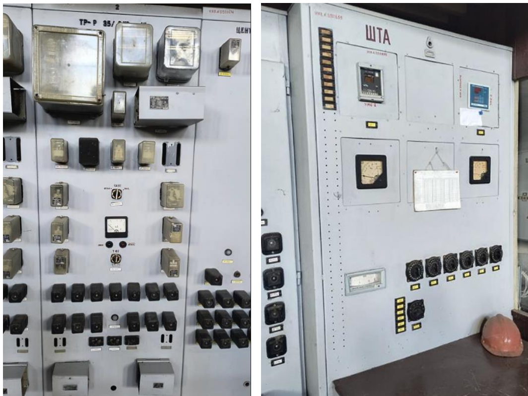
Figure 3-2 Outdated control and monitoring cabinets
