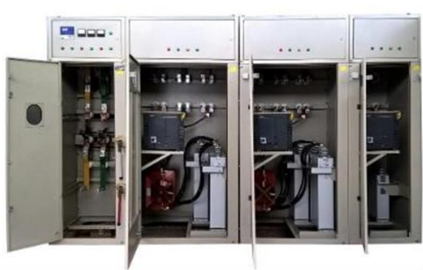
Figure 3-6 Example of 6 kV Capacitor installation
