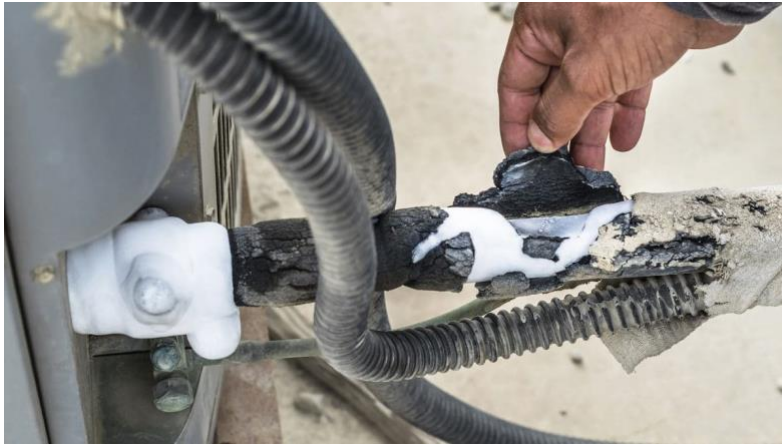
Figure 16: Example of cooling system leaking refrigerant
