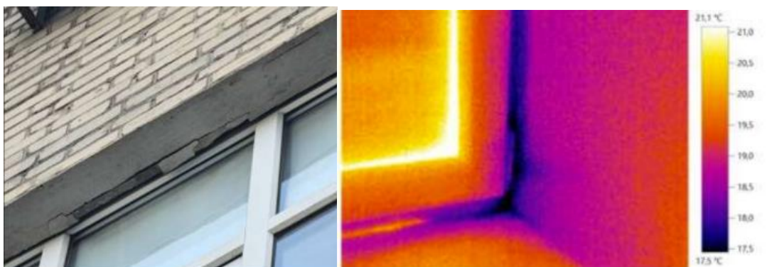
Figure 18: Examples on gaps between exterior wall and window and thermographic image of air infiltration
