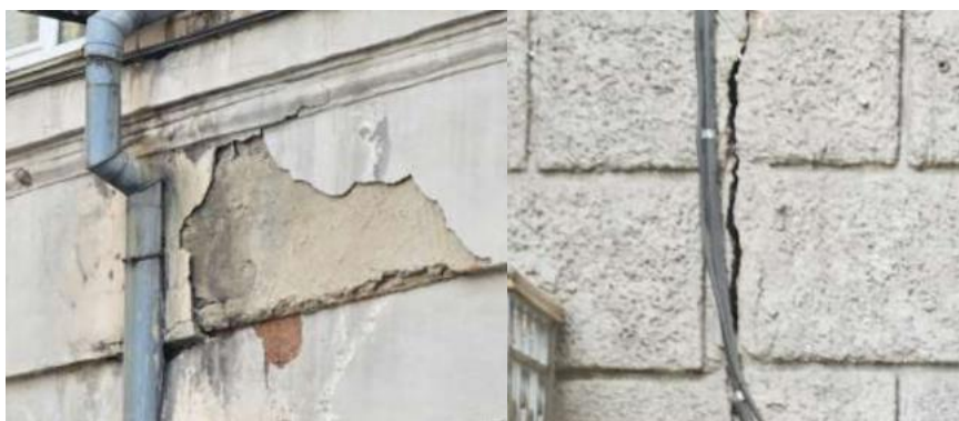
Figure 17: Examples on cracked building façade
